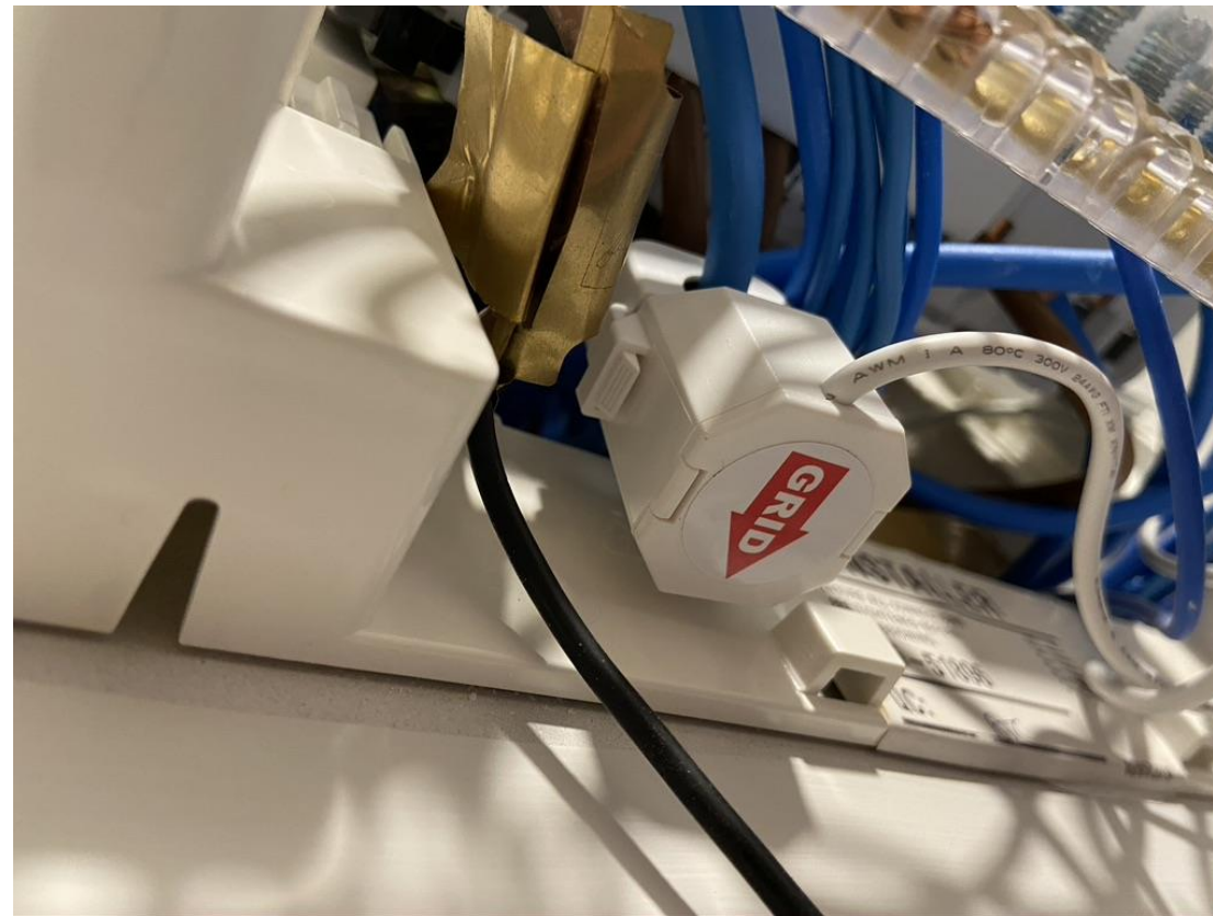
CT + voltage sensor grid mains
